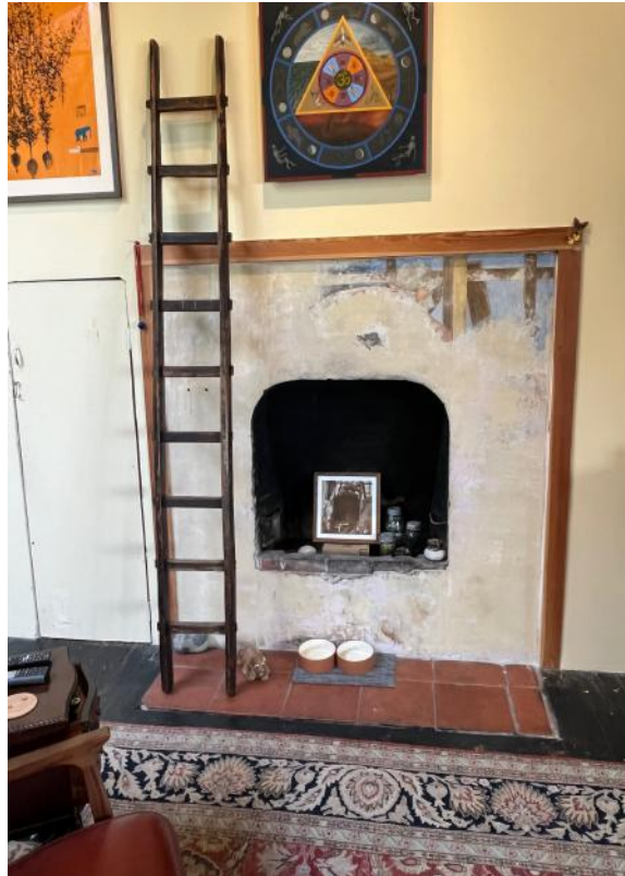
Fireplace at east end of studio space, showing partially-restored John Haley fresco.
