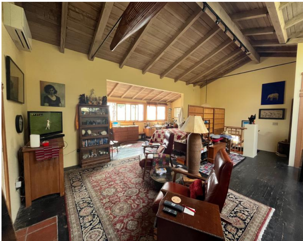
Interior of second floor studio space looking southwest. Wide opening denotes 1938 sleeping porch addition.
